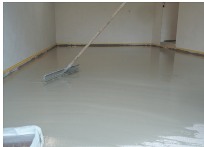
5. Application of the levelling compound Apply the levelling compound ASOCRET-HFF using the squeegee method.
