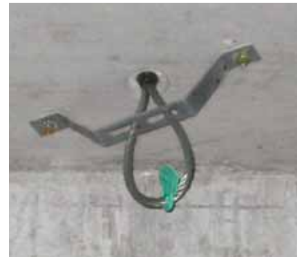
Cable loop installed in a lift shaft
